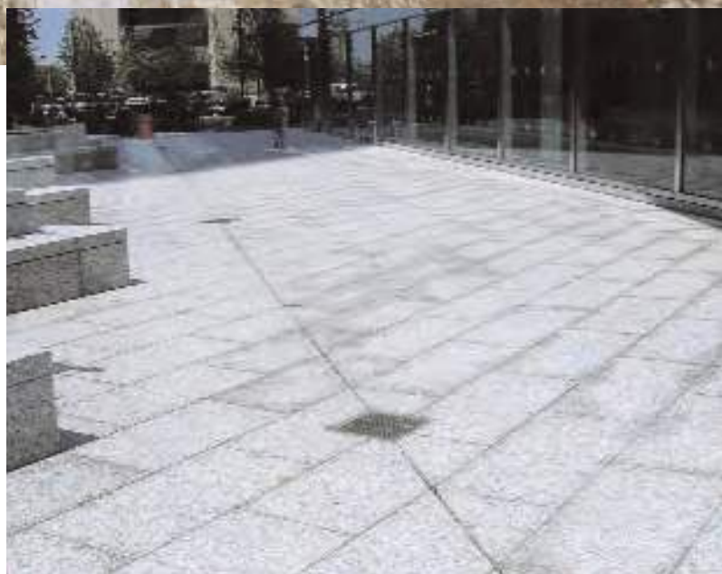
Moisture damage on exterior floor slabs.
